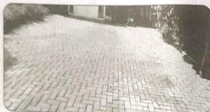
Gaps in concrete surface of road
